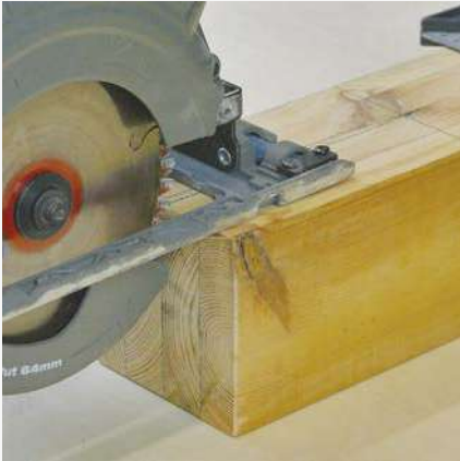
1 Making a cutout in the centre of the post for a recessed support.
