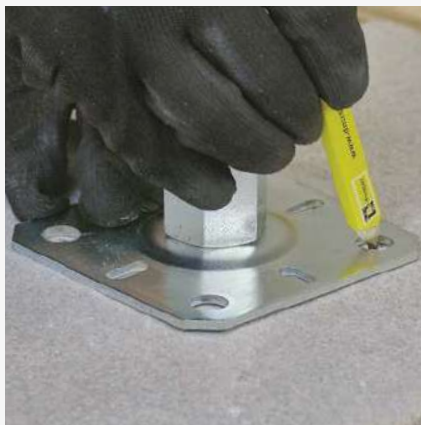
5 Applying the lower support plate and marking out the drilling points in the concrete.
